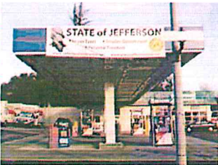
TEMPORARY SIGNAGE ON CANOPY FASCIA
