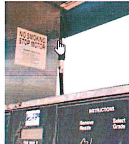
PUMP TOPPER MISSING
